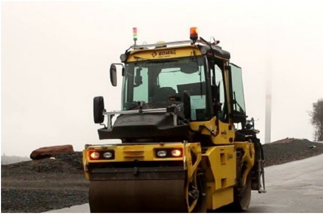
a) Tandem roller performing autonomous asphalt compaction Fig. 9: Examples of off-road robots using behavior networks [11]
